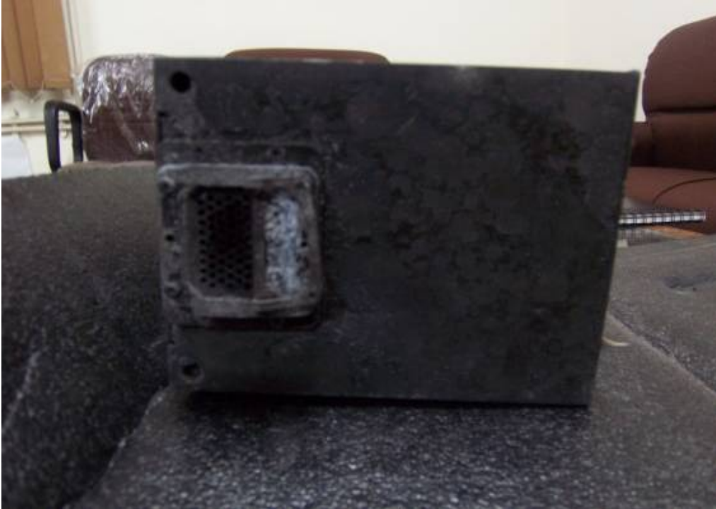
Photo 5: Connector of the CVR Damaged Due to Fire
